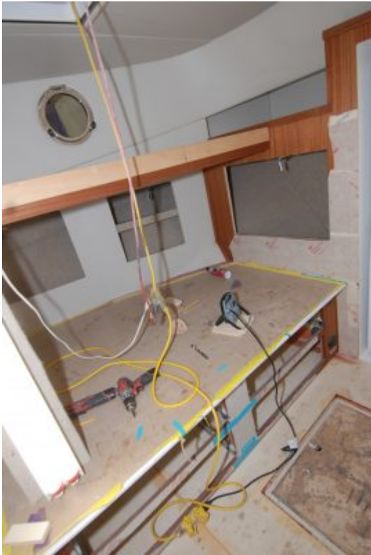
Here is the 2nd stateroom bunks. Ava gets the top, she is so excited!
