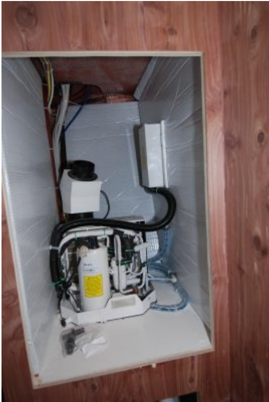
We opted for a small A/C unit that will cool the master stateroom or the pilothouse.
