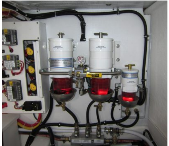
Fuel filtration system.
