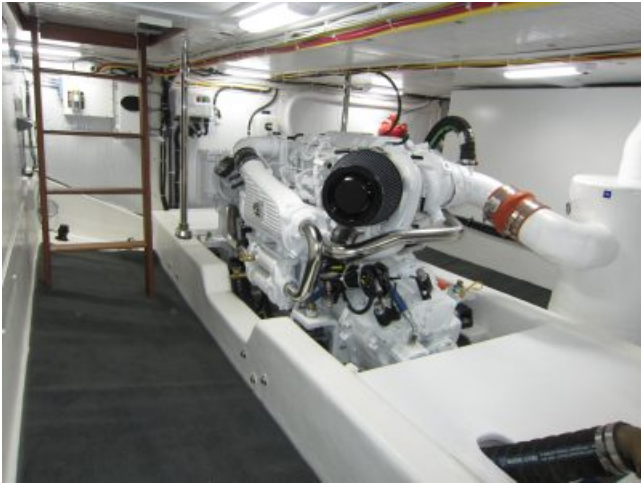
Finished engine room. Clean and organized!
