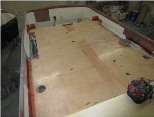
With all the major mechanical installed the salon floor is now installed.
